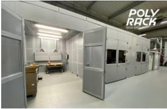
4: Grinding cabins in the new plant 4.
